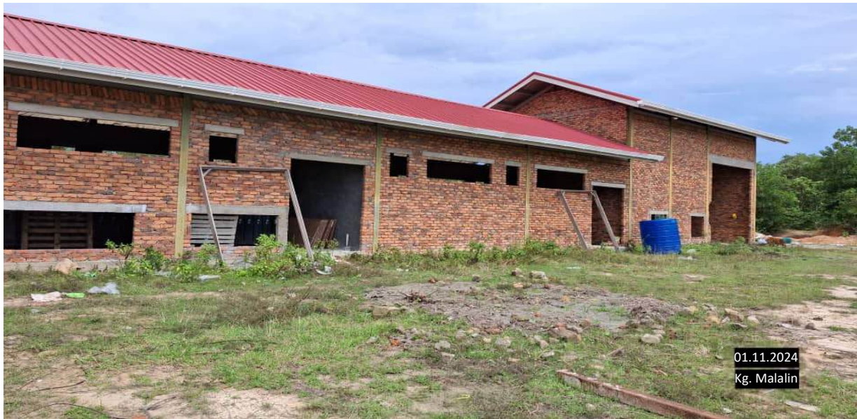
a) Power House Building
