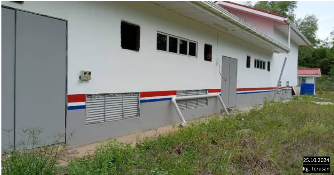
a) Power House Building
