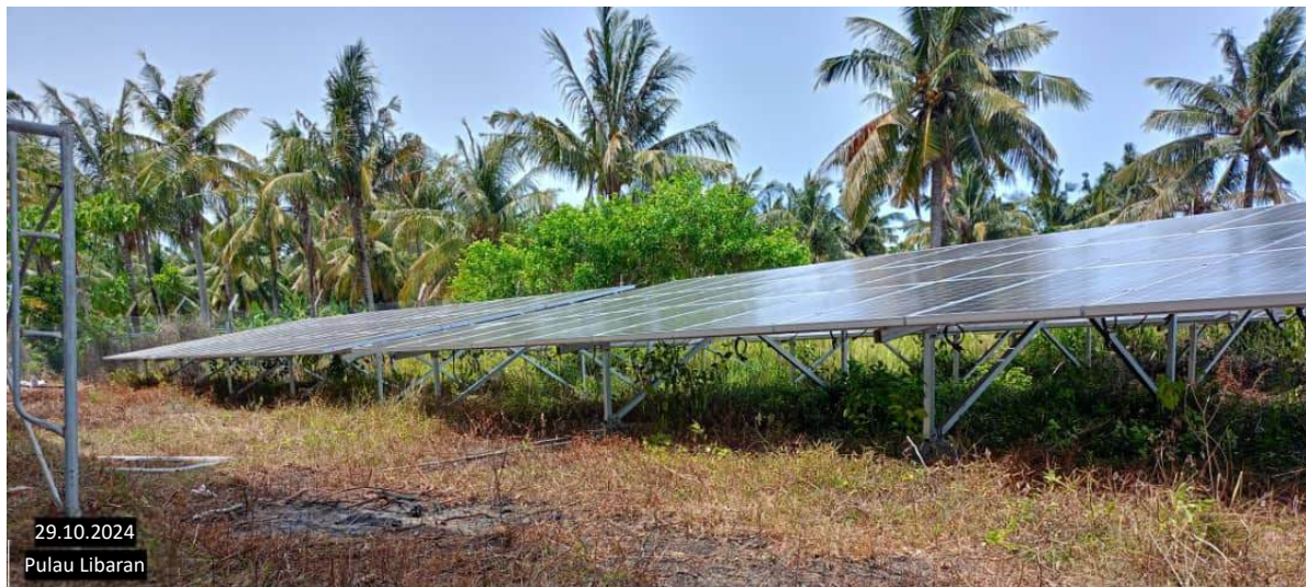
c) Solar Panel
